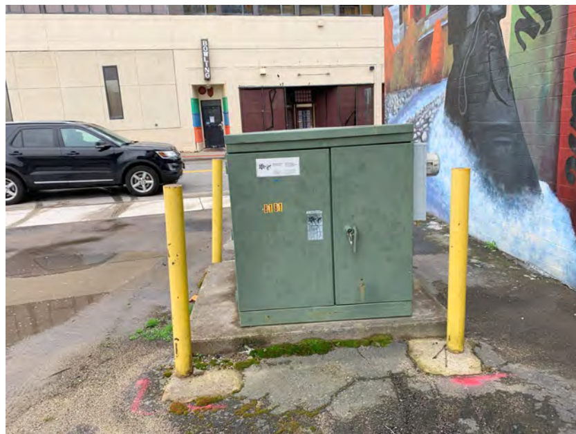
Photo 6 Transformer box just outside of the Site boundary on the abutting parking garage. Southern-abutting parcel.
